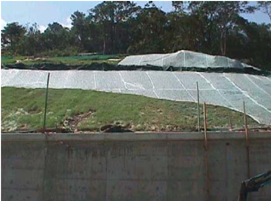
Figure 2: Slope with poor vegetation coverage
